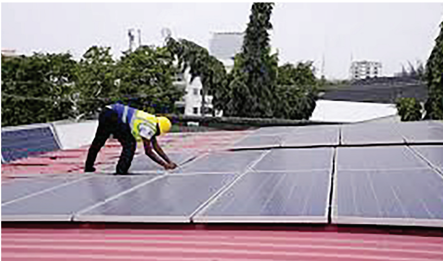
Oladapo Adekunle, an engineer with Rensource Energy, installs solar panels on a roof of a house in Lagos, Nigeria.
